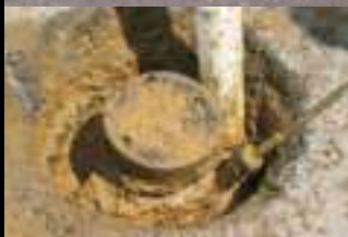
Hydro excavation valve box repair results in a small and less disruptive excavation area.
